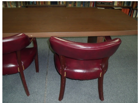
Existing run of carpet found in the chapter house's library. After years of use the carpet has begun to come apart at its seams.
