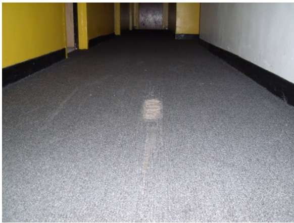
Existing run of carpet found in the upstairs hallway of the Delta Tau Delta chapter house. Note of the wear of the carpet in the center of the photo.
