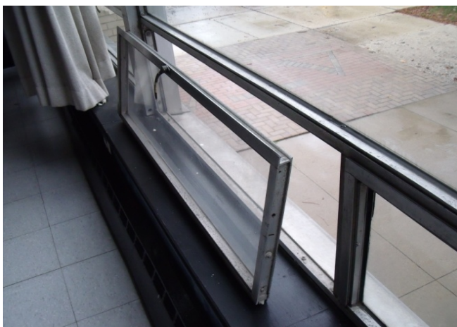
Many of the windows in the building have aged over time, some becoming inoperable. In this picture one inoperable window is shown.
