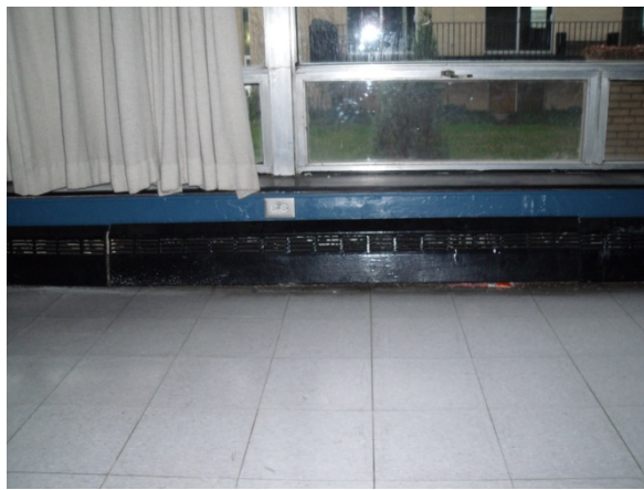
Picture viewing one of the many runs of raditors that around found throughout the building.
