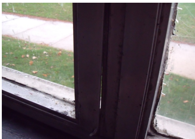
Air infiltration into the structure is one source of high energy costs. Here one can see a visible gap in the windows allowing air to easily flow in and out of the building.
