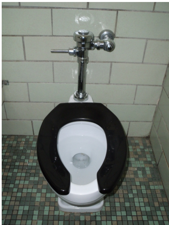
View of current toilet fixture found throughout the DTD house. All toilets found throughout the house use 3.5 gallons per flush.
