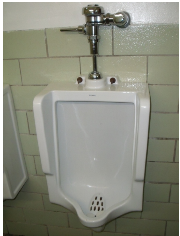
This 1.0 gallon per flush urinal fixture is the current urinal fixture of choice in the building.
