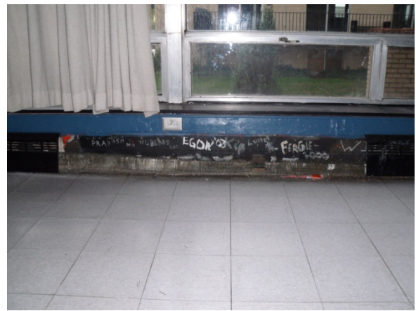
When the cover is removed its easily seen how the many of the fin tubes in the system have been bent or broken thereby hindering the performance of the system.
