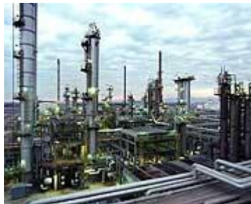
Located just south of Gary, Ind., the Whiting refinery is the second largest of BP's five U.S. refining operations.
