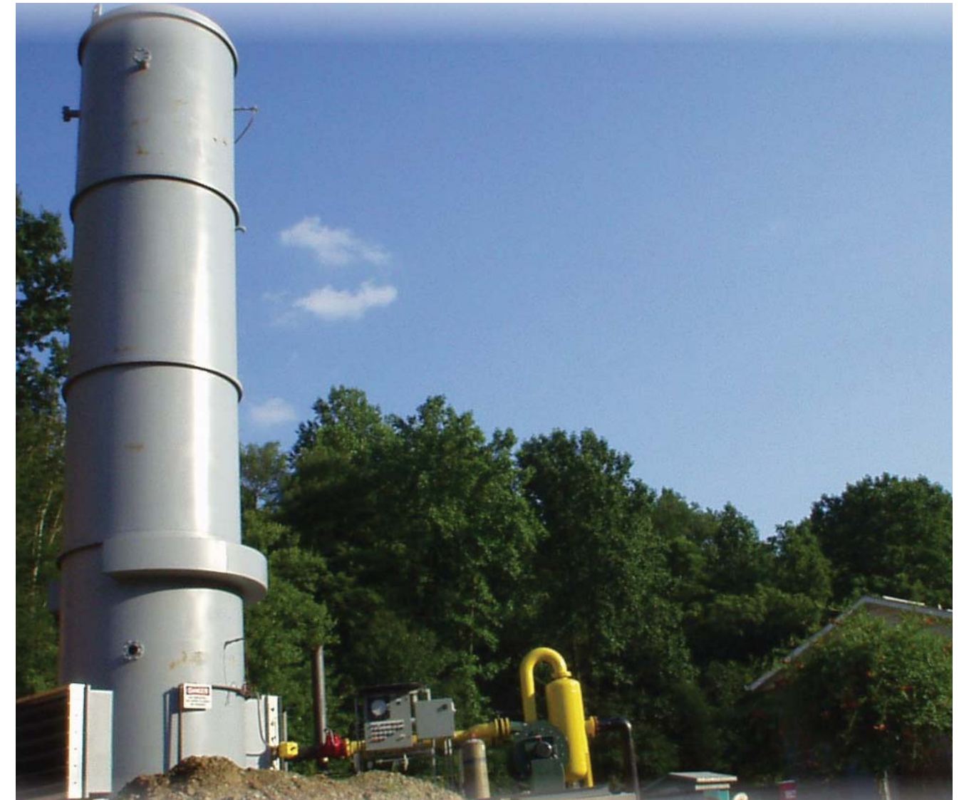
LFG Gas Flares Image Courtesy of MRW Technologies, http://www.mrw-tech.com/landfill_gas_flares.html
