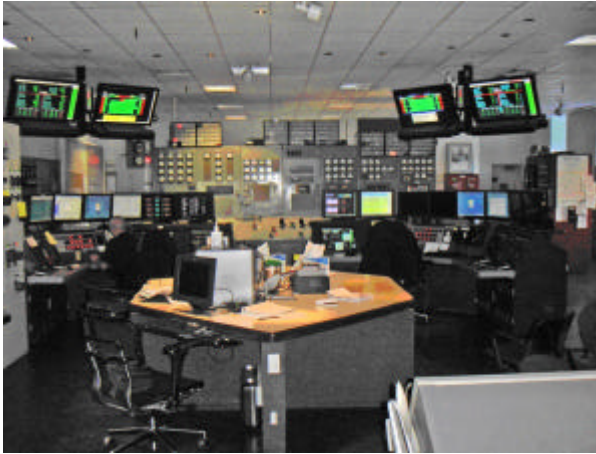
photo of Control Room (Waukegan Plant)
