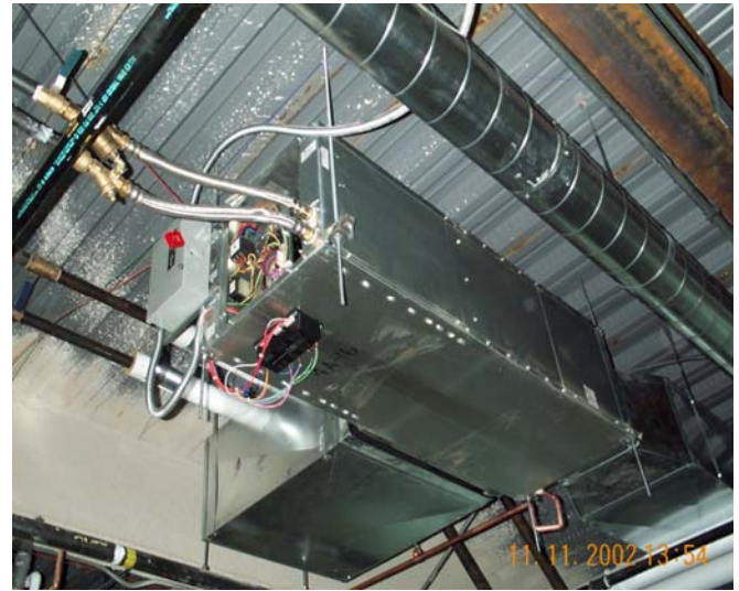
Figure 4. Photograph of a typical horizontal, ceiling-mounted water-air heat pump.
