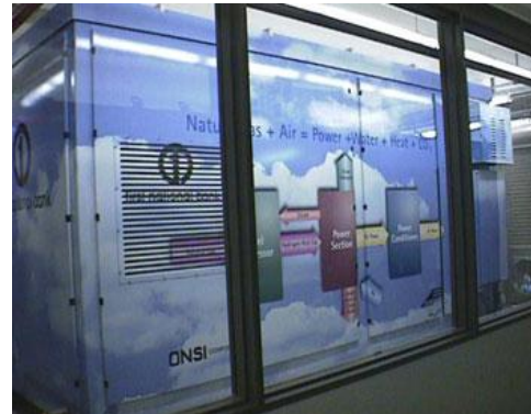
Fuel Cell installation at FNBO
