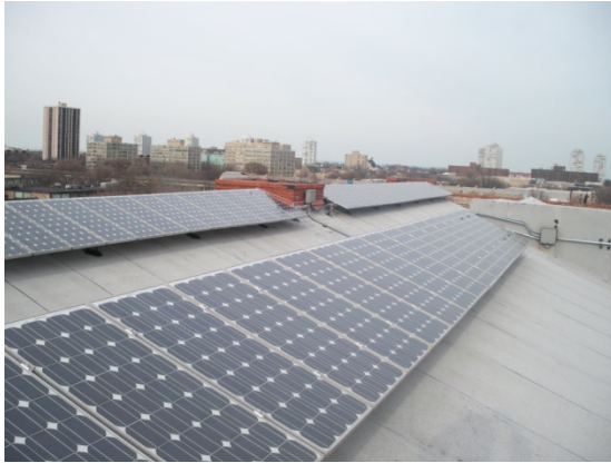
Photovoltaic Panels on the roof of Machinery Hall
