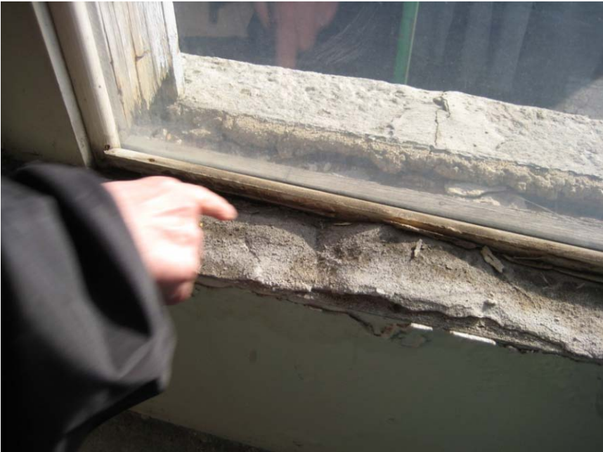
Deteriorating window sill allows air infiltration
