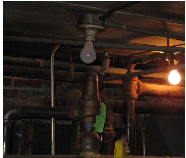
Unnecessary 300 Watt incandescent lamps
