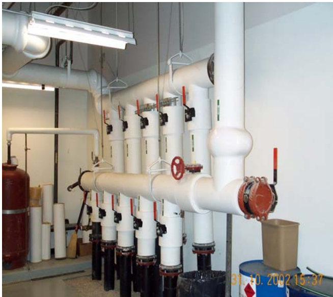
Figure 3. Photograph of the mechanical room at the Canyon View High School, showing the ground loop field supply and return headers.
