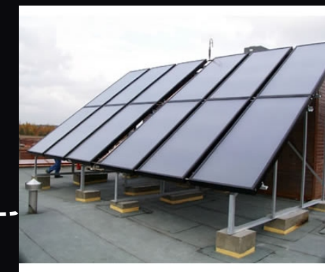
Rooftop Solar Panels
