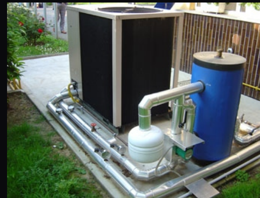
Pipes connected to wall mounted units for making cool air & extra heat goes to kilns - waste heat from kilns directed to chiller for reuse
