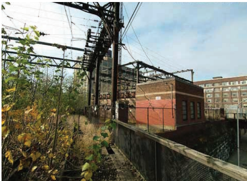
Electrical lines + power station
