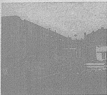
WORKMEN ARE SHOWN preparing to pour concrete for the second floor of the new dormitory, located at 33rd and Michigan. The men say that with warmer weather, construction will proceed rapidly.
