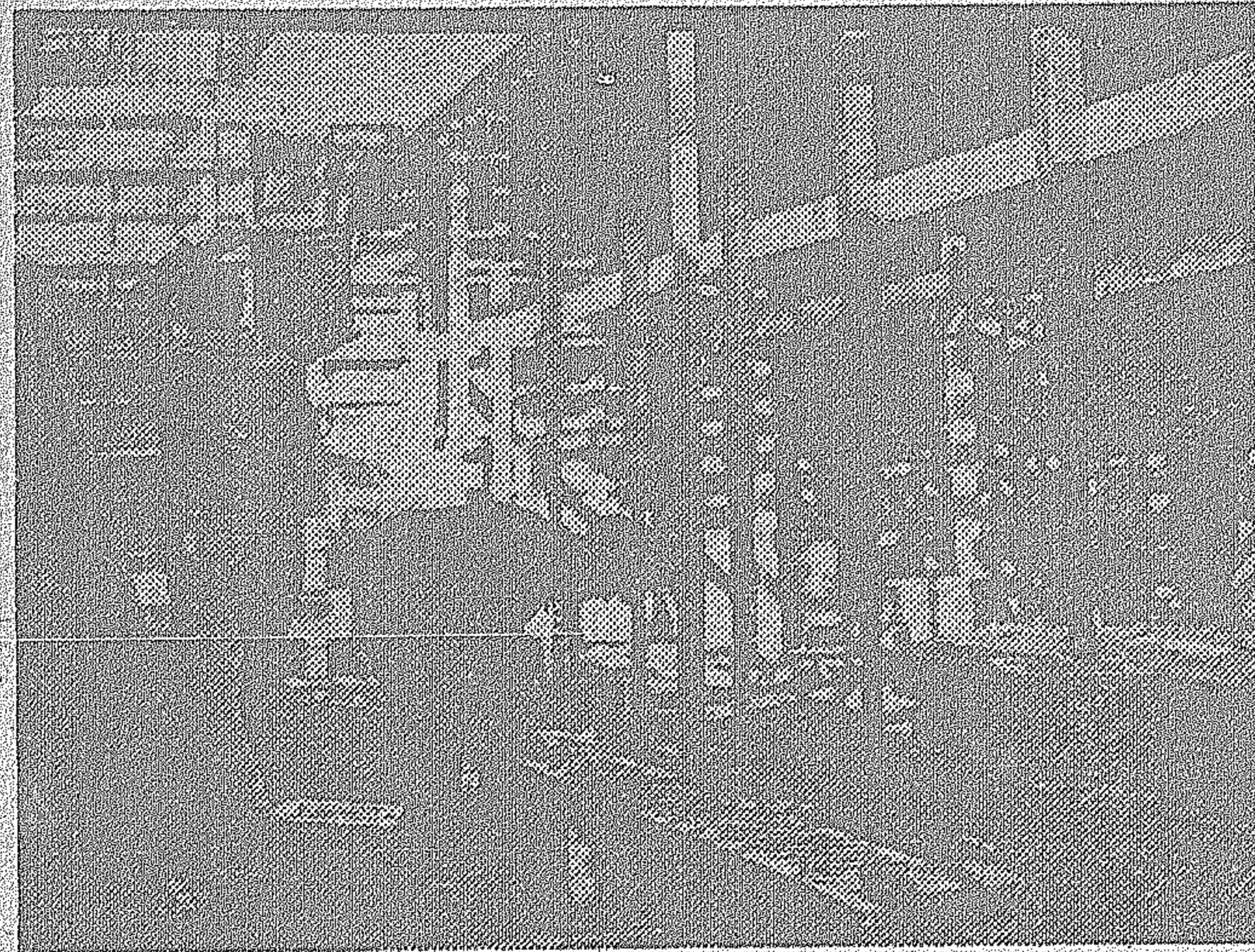
WORKMEN ARE PUTTING in the concrete block wall of the foundation of the new dormitory after 110,000 cubic feet of dirt have been excavated. See story on page 3.
