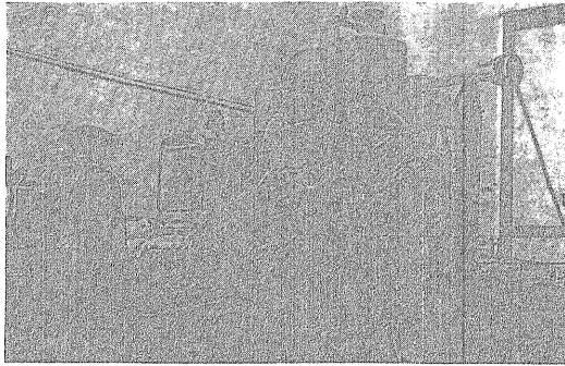
PUTTY-PUTTY —Workmen have been busy spreading concrete for the foundations of the new temporary buildings to be erected on the IIT campus.
