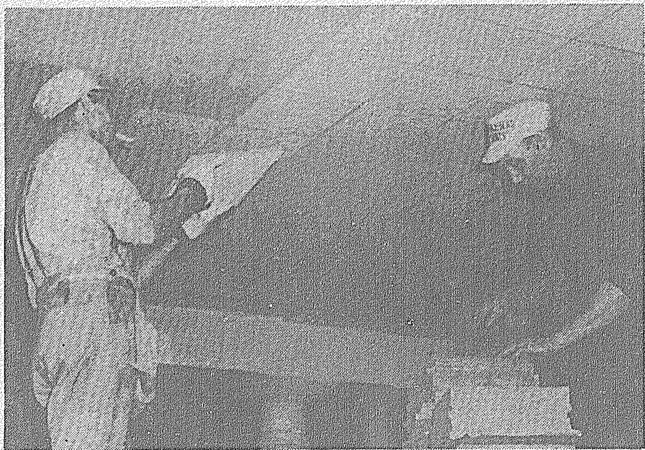
Silence reigns in the Armour cafeteria since the installation last week of a sound-absorbing ceiling.
